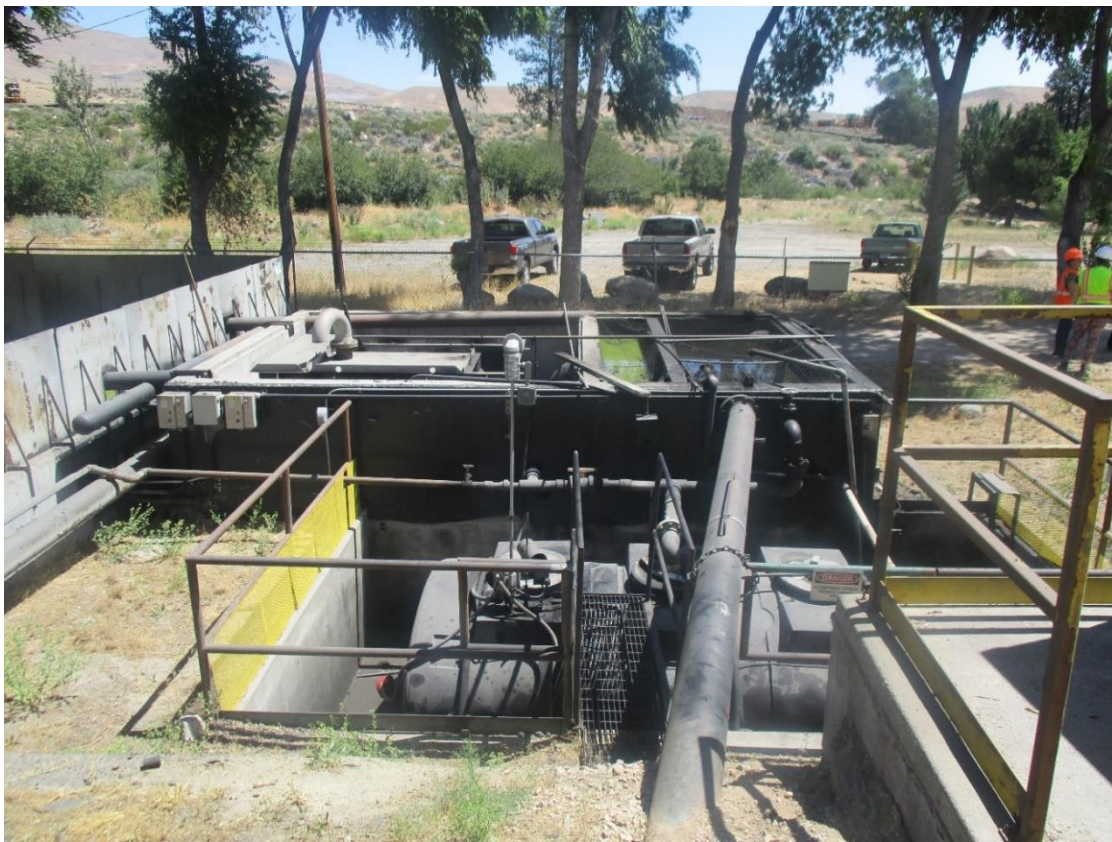
Figure 16 - Oil Water Separators in the background, Waste Oil Tank in the foreground
