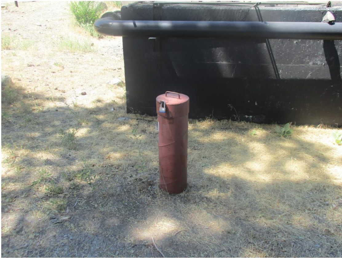
Figure 18 - Monitoring Well 1 East of the Oil Water Separators
