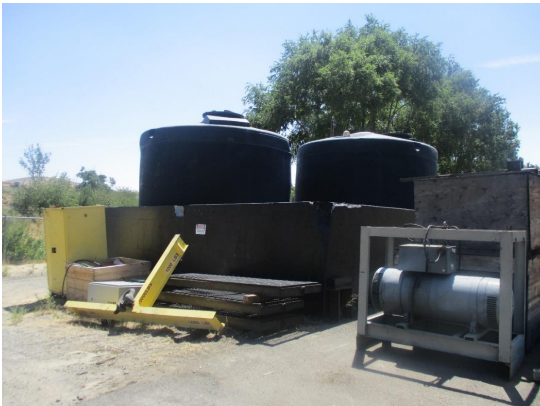
Figure 15 - Two 10,000-gallon storage tanks within concrete secondary containment
