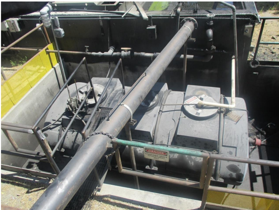
Figure 17 - Waste Oil Tank
